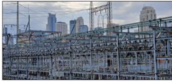
Figure 2. Xcel's power plant structure is located on the pier of the old Pillsbury Mill next to SAFL. (John Foley)
