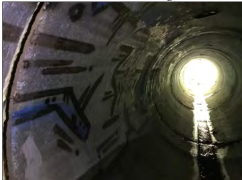
Figure 11a. The Highland Creek tunnel with its curious “prehistoric cave art” graffiti.
