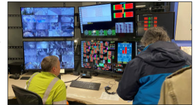
The control room
