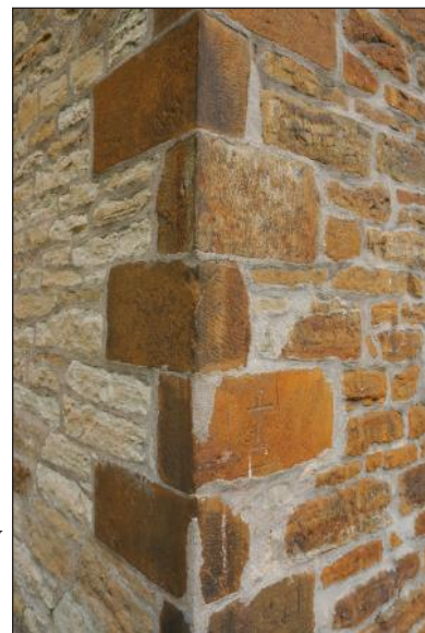
Stones on the Faribault House are still solid after 185 years. The stones have been repointed
