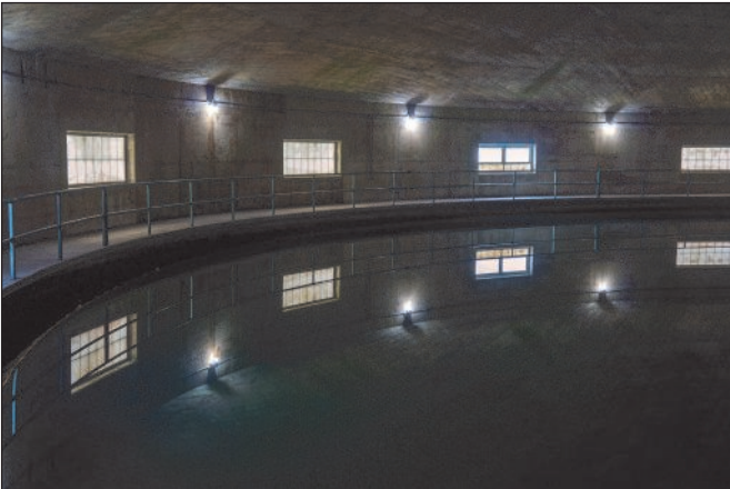
Round clarifier tank
