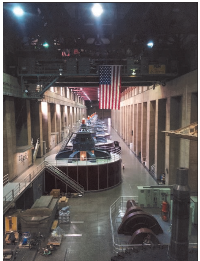
Generators in Hoover Dam
